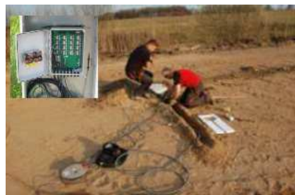
Figure 3: Details of the installation test site, pressure & temperature data recorder.
